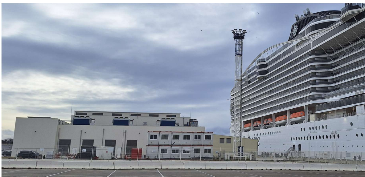
The cruise terminal substation at the Léon Gourret Terminal in Marseille, handling three simultaneous connections. View from the north
