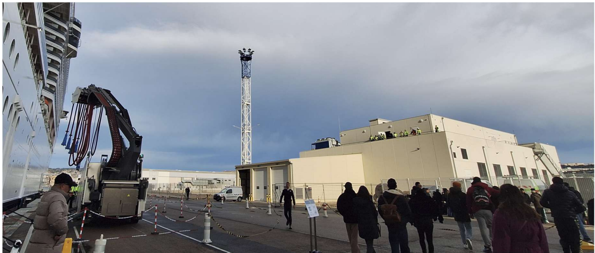
The cruise terminal substation at the Léon Gourret Terminal in Marseille, handling three simultaneous connections. View from the southwest
